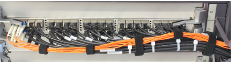
Figure 6-121 Arrangement of optical fibers and SFP+ cables
