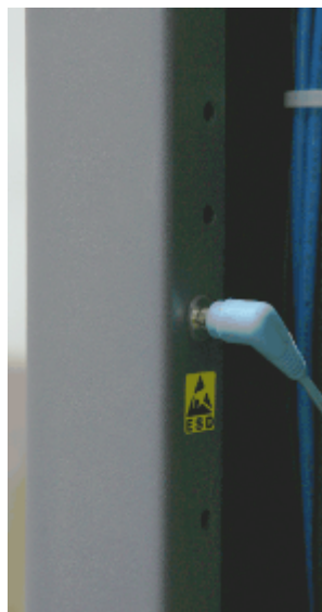
Figure 1-10 ESD jack in the middle of the N68E cabinet
